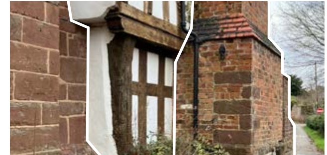
Figure 45: Churton Hall well-demonstrates Churton's building material mix of red sandstone, red brick and timber framing.
